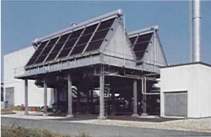
Figure 2.15: Example of an air-cooled condenser for condensation of turbine exhaust steam [tm111, BDAG, 1996]
