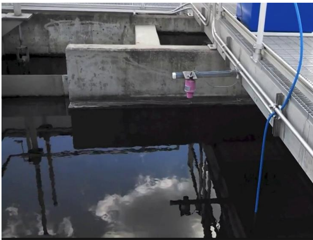
Figur 9-1 Eksempel: Ultralydssensor placeret over vandspejlet i et spildevandsbassin (Kilde: https://store.aquatechnologygroup.com/products/nivelco-easytrek-sp-300-series-compact-ultrasonic-transmitter/#gsc.tab=0 )
