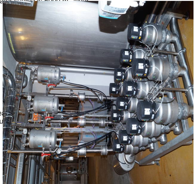
Pump seal water system installed at Them Dairy (Copyright photo Them Dairy)
