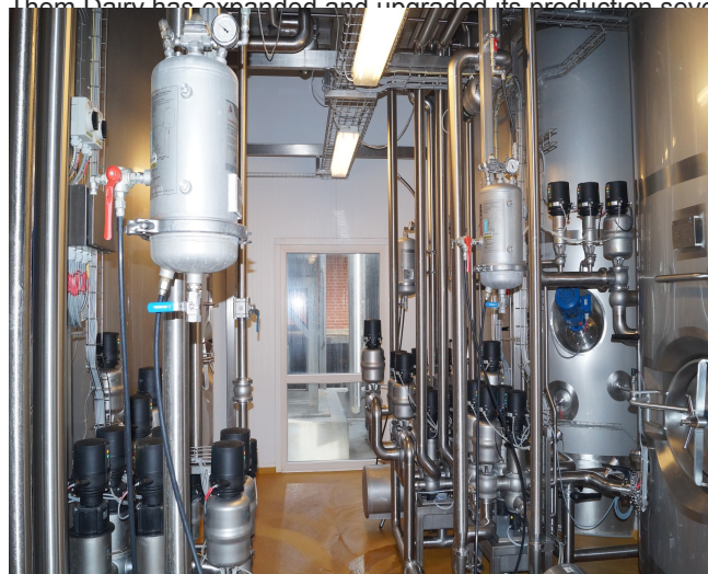
New Cleaning in Place (CIP) system installed at Them Dairy (copyright photo Them Dairy)
